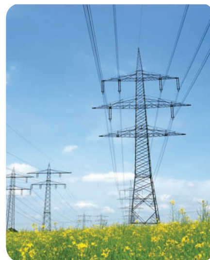
▲ Electricity cables: aluminium (light) with a steel core (strong).
